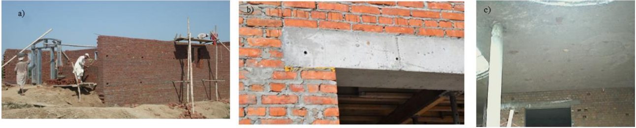
Figure 2. a) Construction process and structural detailing b) lintel and wall bonding view, and c) poor quality of RC slab construction, bricks are added in RC roof-slab (Ali, 2006 )
